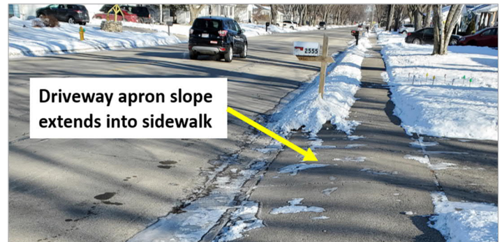
Example of driveway apron slope extending into sidewalk through the driveway creating non-compliant cross slopes. Wider terraces and depressed sidewalk profiles will improve these slopes making them ADA compliant.
