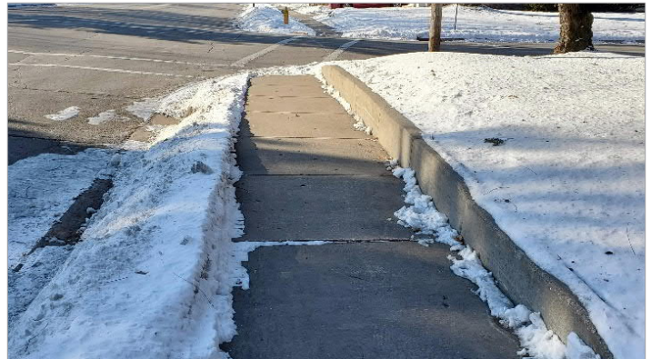
Example of short retaining wall at back of sidewalk to minimize right-of-way impacts north of Simonet Street.
